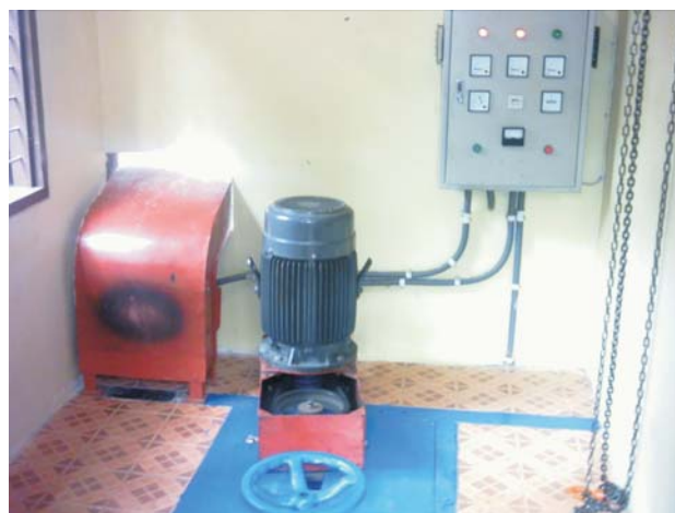
Photo 1. Open Flume Propeller Turbine with ELC in the background installed in the Leuwi Kiara MHP, Tasikmalaya Regency, West Java. The equipment was manufactured and supplied by CIT and HPT, Bandung.
