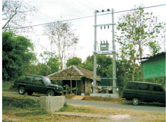
Photo 2: The scheme is inter-connected at medium voltage (20kV). The transformer and inter-connection point is located directly at the road side approximately 150m from the power house
