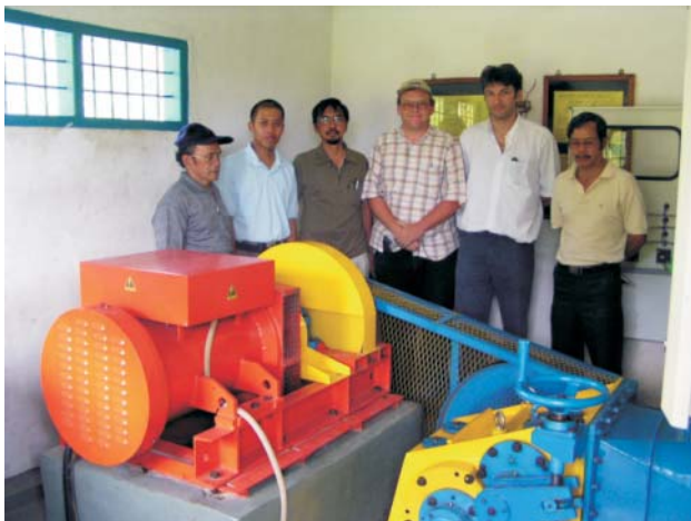
Photo 1: Representatives from JASTEK, GTZ-MHPP, PLN Mojokerto and PT. Heksa Prakarsa Teknik in the power house of the 25kW Kali Maron scheme. The plant is the first small private renewable energy project to be commissioned following the introduction of the ministerial decree in June 2002. (PSK TERSEBAR-KEPMEN No: 1122K/30/MEM/2002)
